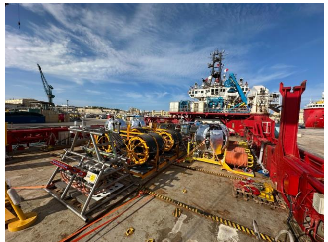
Components for ARCA on the deck of the Optimus Prime ship: in the foreground a junction box, behind it a couple of spools with the submarine interlink cables plus some DUs.
