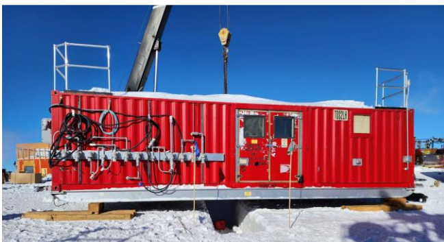
Positioning TOS2 over the trench to allow access to the skis and remove compacting snow inside the skis. (K. Studt, IceCube / NSF)
