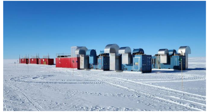
View of Seasonal Equipment Site showing the 3 generators, 3 out of 4 Main Heating Plants, and a Water Tank. (K. Studt, IceCube/NSF)
